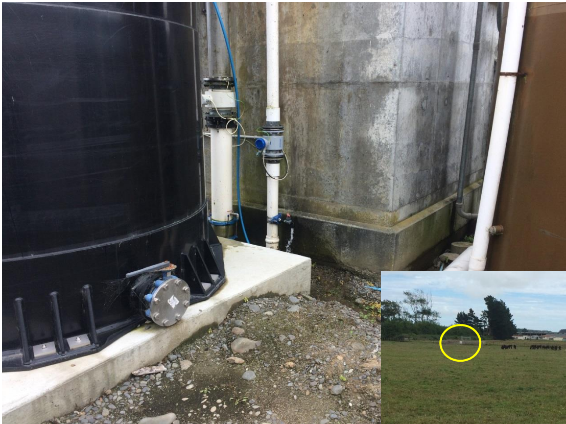
Photograph 2: Bore 5 (OHA_ADJ_GW38) Tap Sample. Bore 5 is located within the paddock across the treatment plant approximately 150m (inset photograph).
