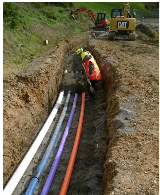
Above: Installation of the PE water pipe and service conduits to the bore.
