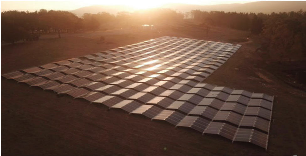
Figure 5 Example of an ‘LMS Energy’ landfill solar system 34
