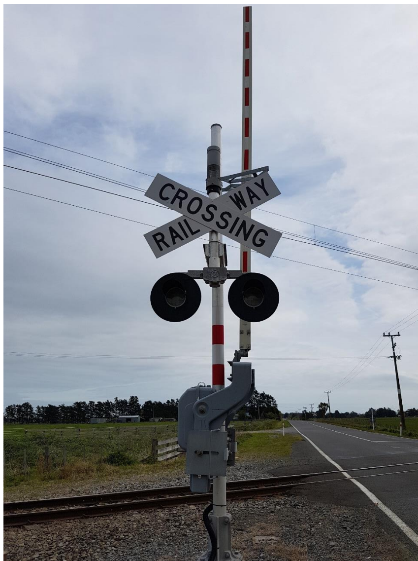
Figure 8: East Approach – Flashing Lights Bells and Half Arm Barrier
