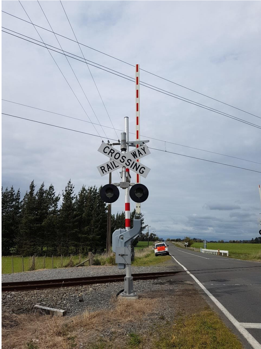
Figure 14: West Approach – Flashing Lights Bells and Half Arm Barrier
