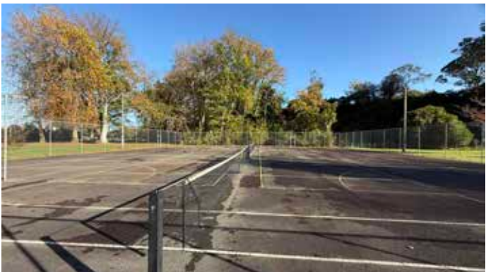
Tennis nets in poor condition
