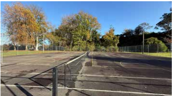
Tennis nets in poor condition
