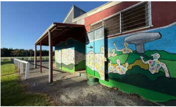
Public toilets and changing room close to car parking. Toilet does not have an accessible access.
