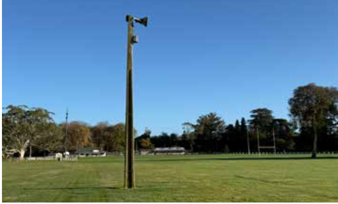
Sports field lighting.
