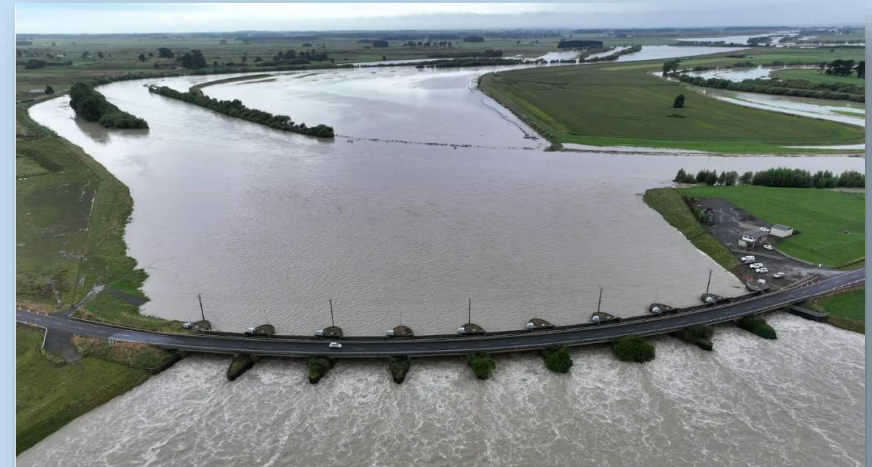
Moutoa floodgates were built in 1962 and are getting a few improvements this year.
